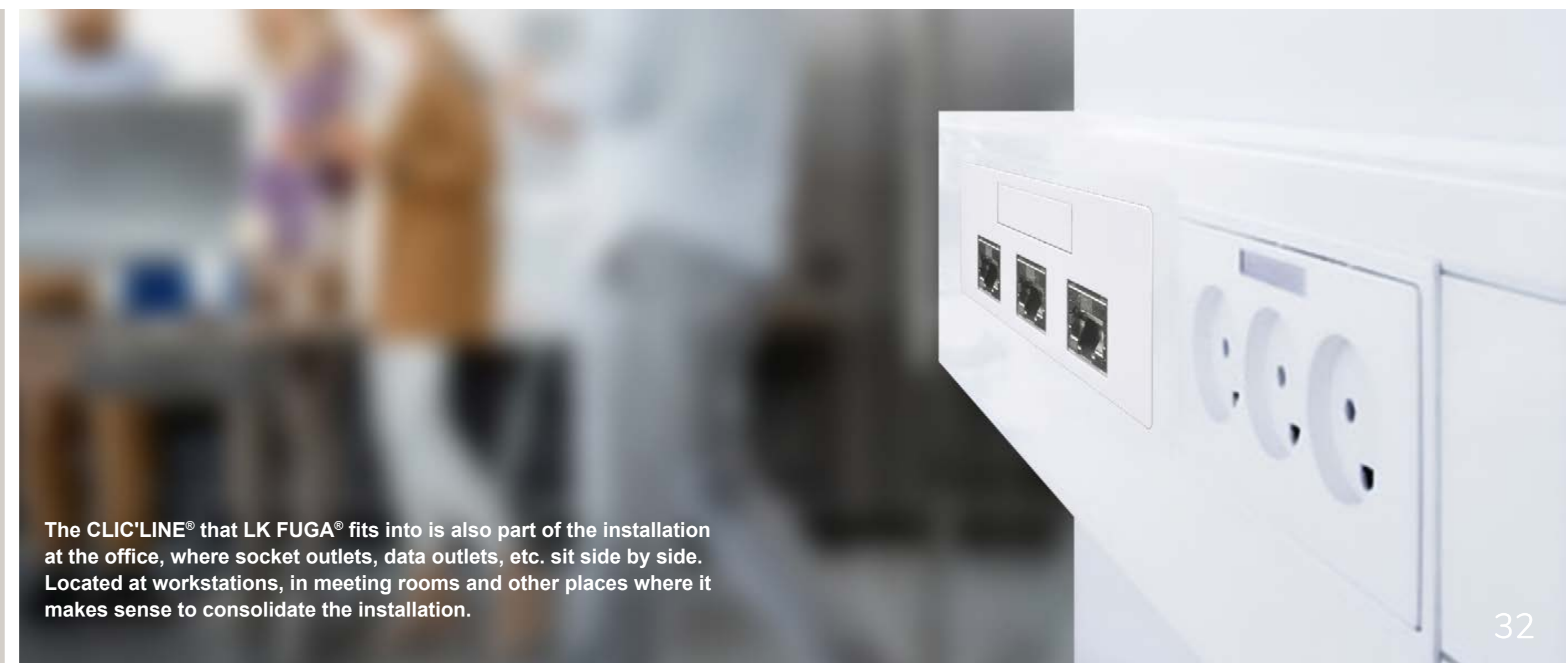
The advertising agency in Copenhagen has a full LK FUGA® solution installed in their office with basic solutions and more advanced features.
